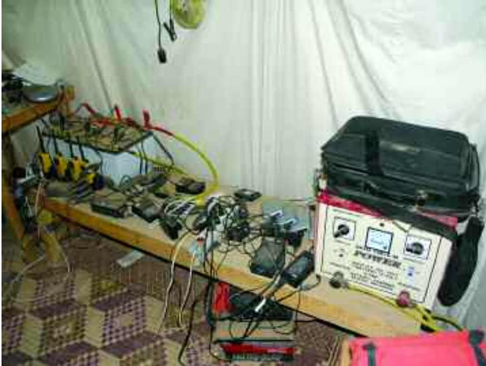
Figure 2. Power station for the ASPS project (Abydos, Egypt). To the right is a 12v battery charger that can be configured to charge up to five car batteries. To the left are a set of car batteries wired in parallel. A power inverter (the circular object in the upper left) is used to generate 220v for the power strips seen in the photo. The remaining items (IPaq computers, walkie-talkies, and rechargeable AA batteries) are charged directly from 12V.
